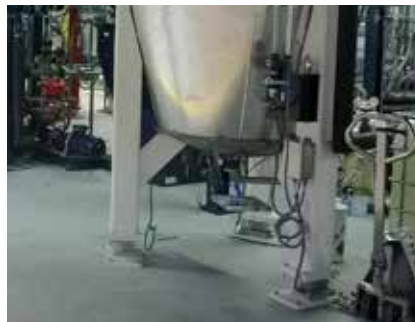
Machine on load cell system
